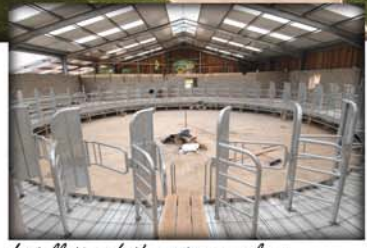
Installation of the rotary parlour
